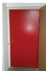
Fire Rated Electrical Shaft Door
