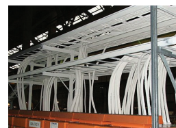
Fire Rated Cable Coating
